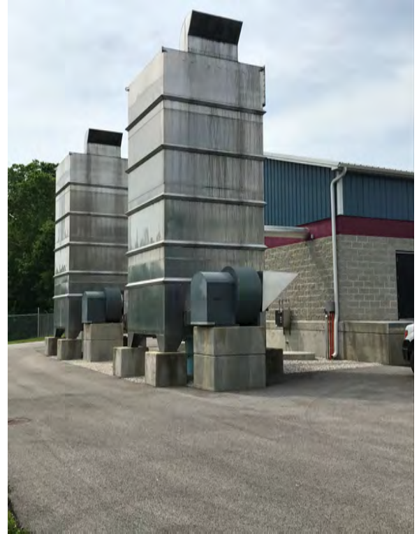
Air Strippers for the removal of the VOC chemical Tetrachloroethylene "PERC"
