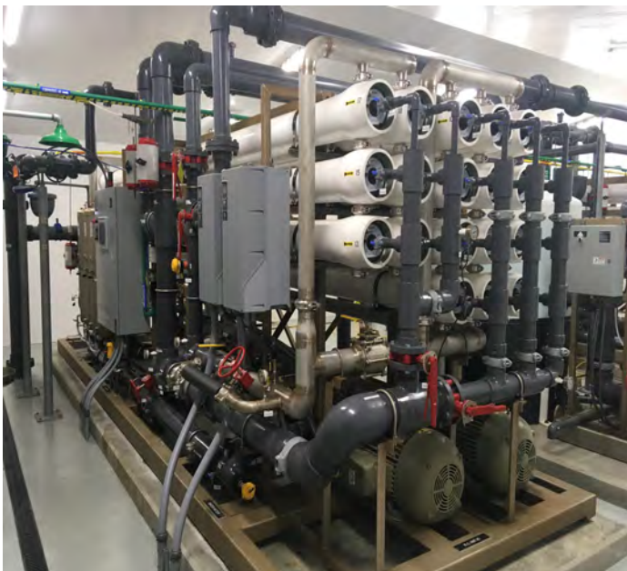
Reverse Osmosis 1,000 GPM Water Treatment
